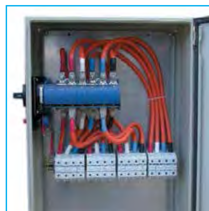
Enclosed & Wired to Terminals
